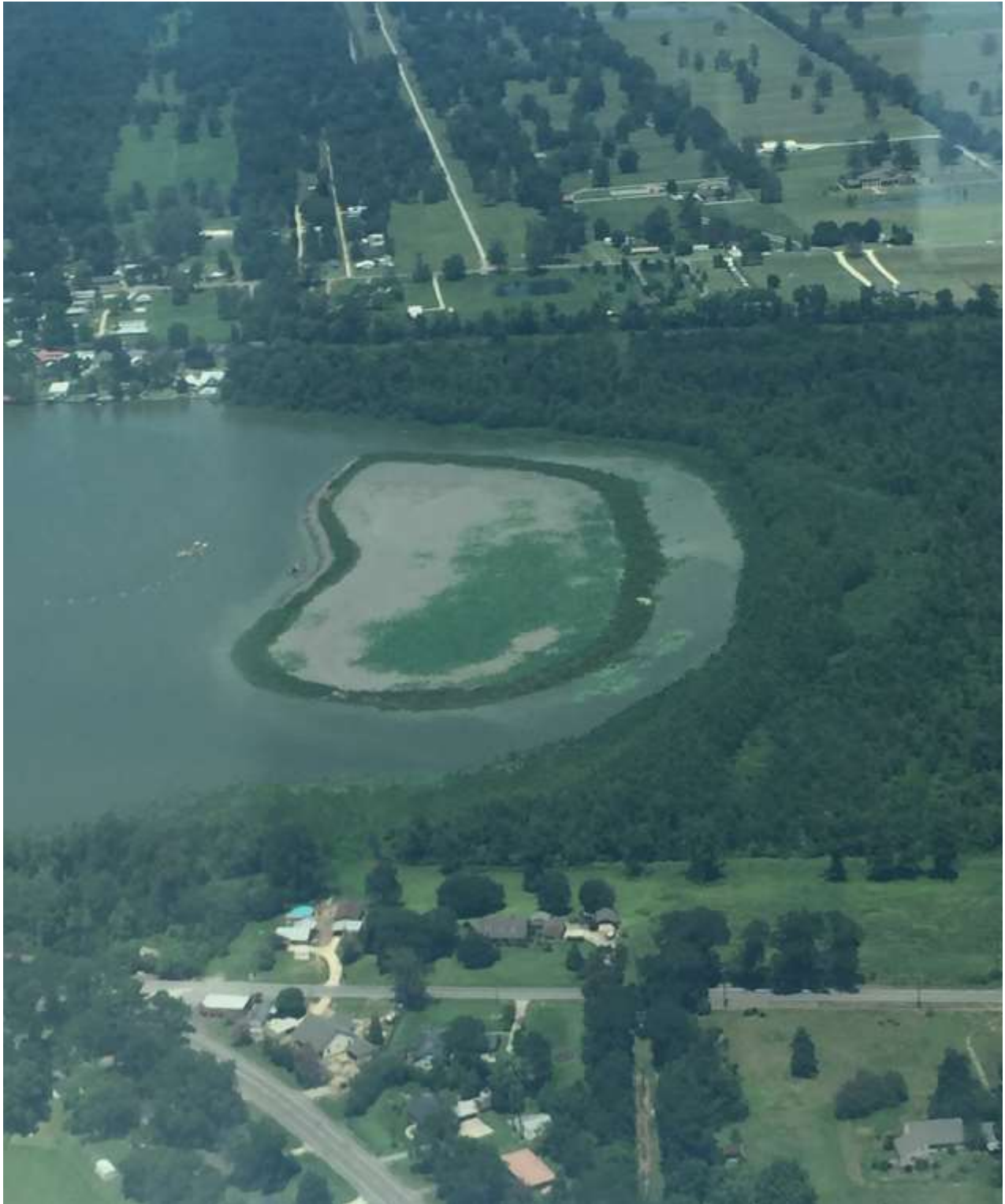
Figure 29: South Flats Island nearing completion. (Source: Photograph taken 8/13/15 courtesy of Randy Boyd, RLB Contracting Inc.)
